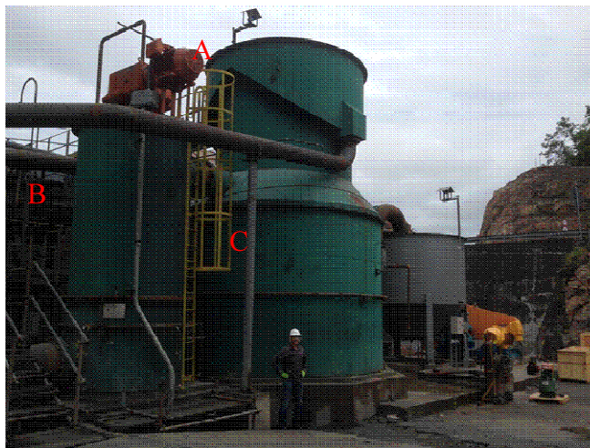
Figure 8 – Installation of Staged Flotation Reactor (SFR) in an operation, showing locations of A) froth recovery (FU), B) particle collection (PCU), and C) bubble disengagement (with permission from Woodgrove technologies)
